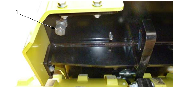
Fig. 9-5 Diesel drain, rear left on chassis
